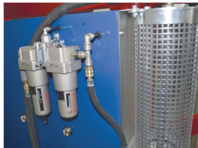
Fuel quality control unit & processing unit
